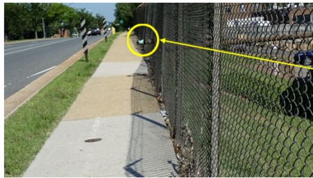
Fire Department Connection
